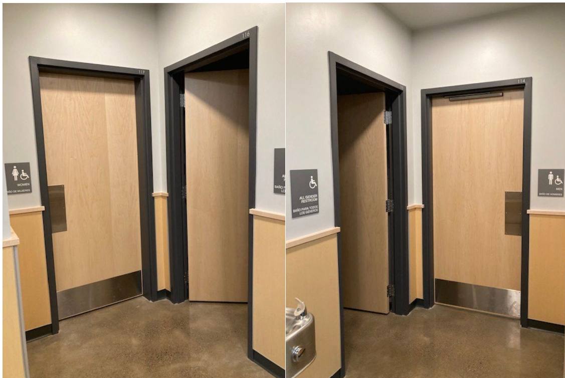
Photo of bathroom entrances/water filling stations
