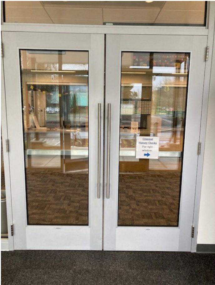
Photo of second set of doors to lobby and inside of the entryway area
